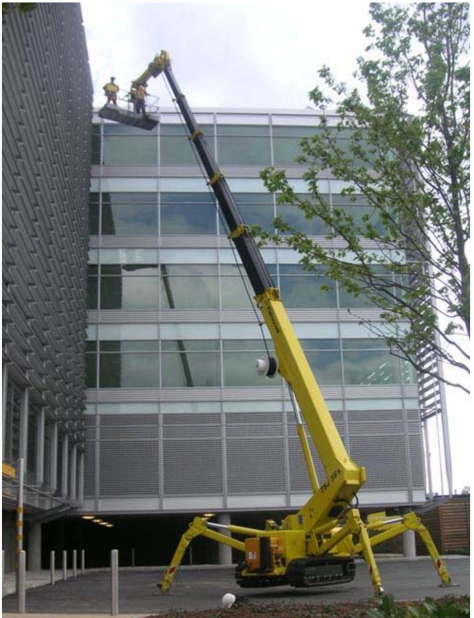
A Palazzani TSJ38 recently sold to 'Enjoy Work' for cleaning and maintenance work at Chiswick Park.
