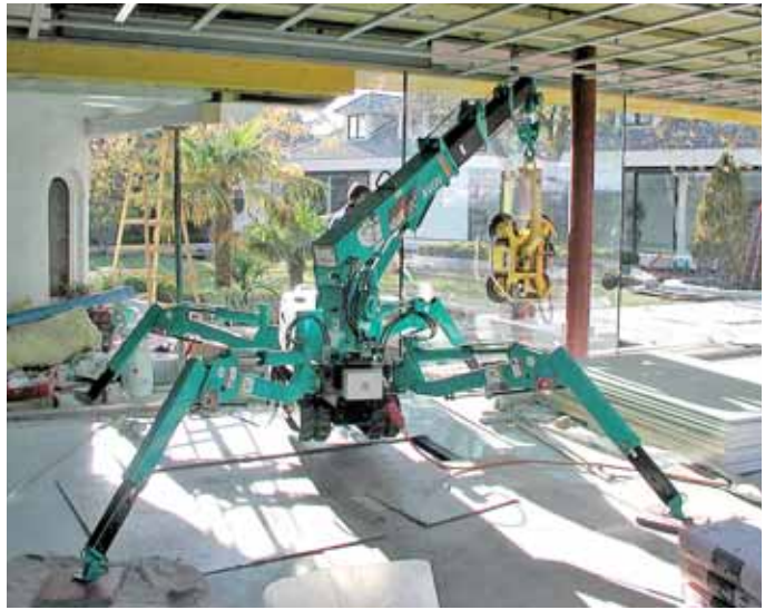
This Maeda mini spider crane shows how it can operate inside the confines of a building to help install glass panels – an application that has established these versatile machines in the UK.
