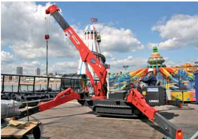
The small size and low ground bearing pressure of this Unic URW-506 allowed it to access the end of Brighton Pier to help erect a new ride.
